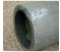
When surface damage prevents a reliable external seal
