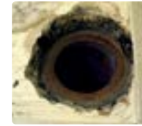
When a pipe is sheared close to a surface, with no stub or spigot
